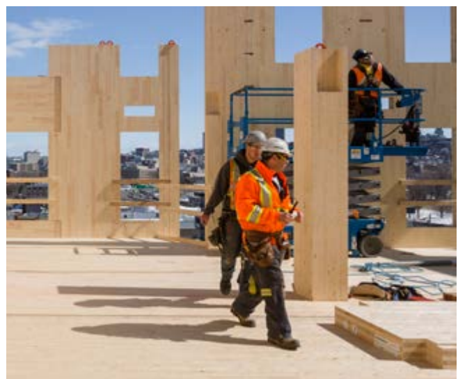
Construction of the 13-storey Origine tall wood building in Quebec City, using mass timber.
