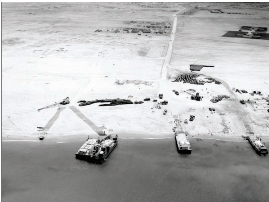
Early airfield construction at Tuy Hoa, Republic of Vietnam, in 1966, with equipment and supplies brought in over the beach. In just one year's time, airmen engineers transformed isolated real estate to the fully operational Tuy Hoa AB. U.S. AIR FORCE PHOTOS
