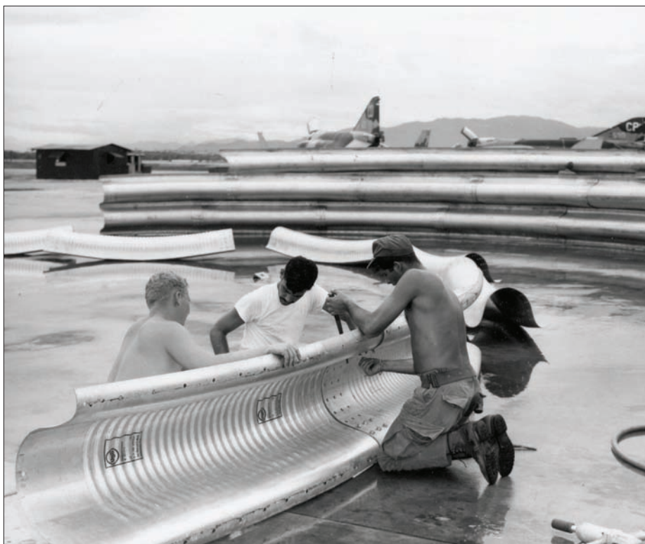
Members of the 820th Civil Engineer Squadron RED HORSE belt together panels of galvanized steel to make an arch for an aircraft shelter under construction at Da Nang AB in South Vietnam, October 1968.
