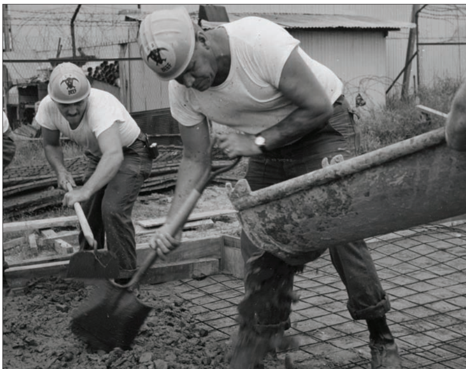
(Top) A RED HORSE crew operates quarry equipment at Tuy Hoa AB, South Vietnam, in 1966. (Bottom) Airmen with Prime BEEF pour concrete for the floor of a building at Tan Son Nhut AB in South Vietnam.
