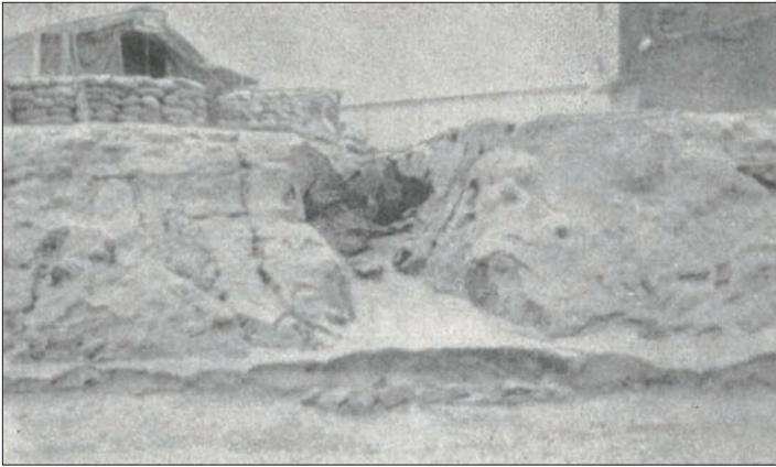
Figure 1. Erosion of Unprotected Ditch Banks.
