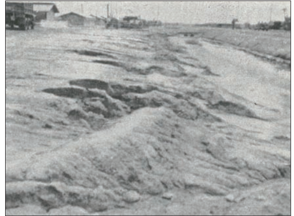
Figure 4. Erosion of 1:5 Slope
